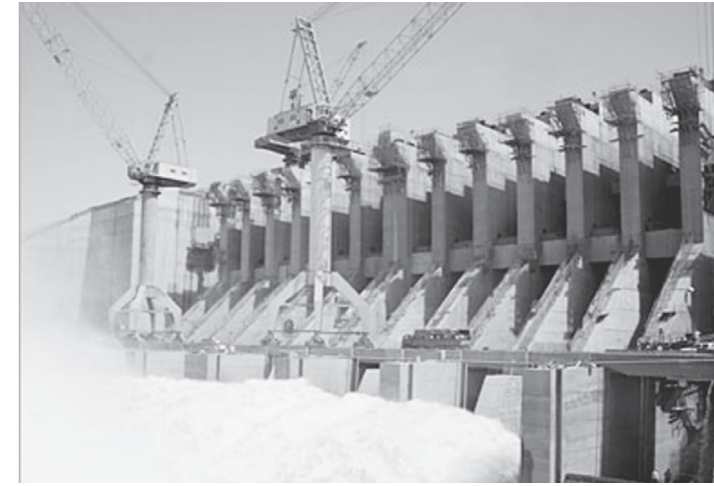
Electricity: Built on the Nile's fourth cataract, the Merowe Dam in northern Sudan is the largest contemporary hydropower project in Africa. EMBASSY OF SUDAN
