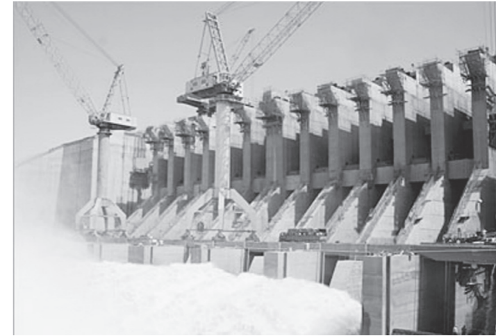
Electricity: Built on the Nile's fourth cataract, the Merowe Dam in northern Sudan is the largest contemporary hydropower project in Africa. EMBASSY OF SUDAN
